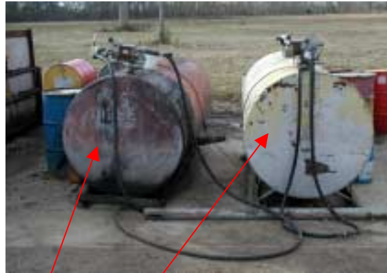
Diesel and gasoline tanks at the Leonville maintenance yard
