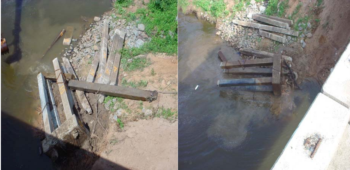
Above photographs were supplied by DOTD and show pieces of bridge at Twelve Mile Bayou removed by Specialized Response Solutions.
