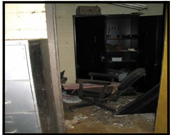
Existing Unusable Office at Research Farm
