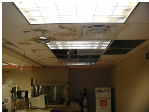
Exhibit 15: Mold in A. O. Williams Hall
