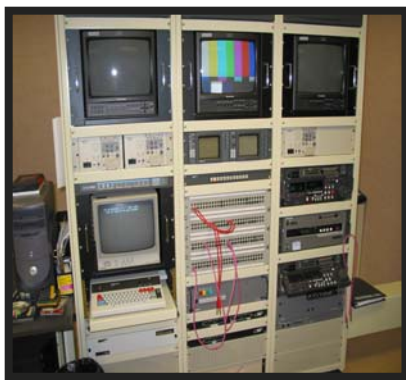
Example of Untagged Equipment in SUAREC Television Studio
