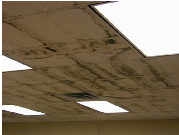
Exhibit 10: Mold in A. O. Williams Hall
