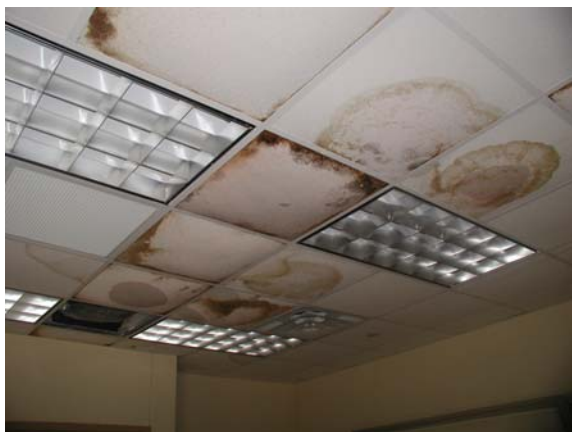
Exhibit 14: Mold in A. O. Williams Hall
