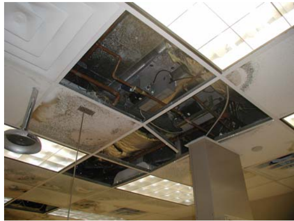
Exhibit 11: Missing Tiles Because of Moisture Problems in A. O. Williams Hall
